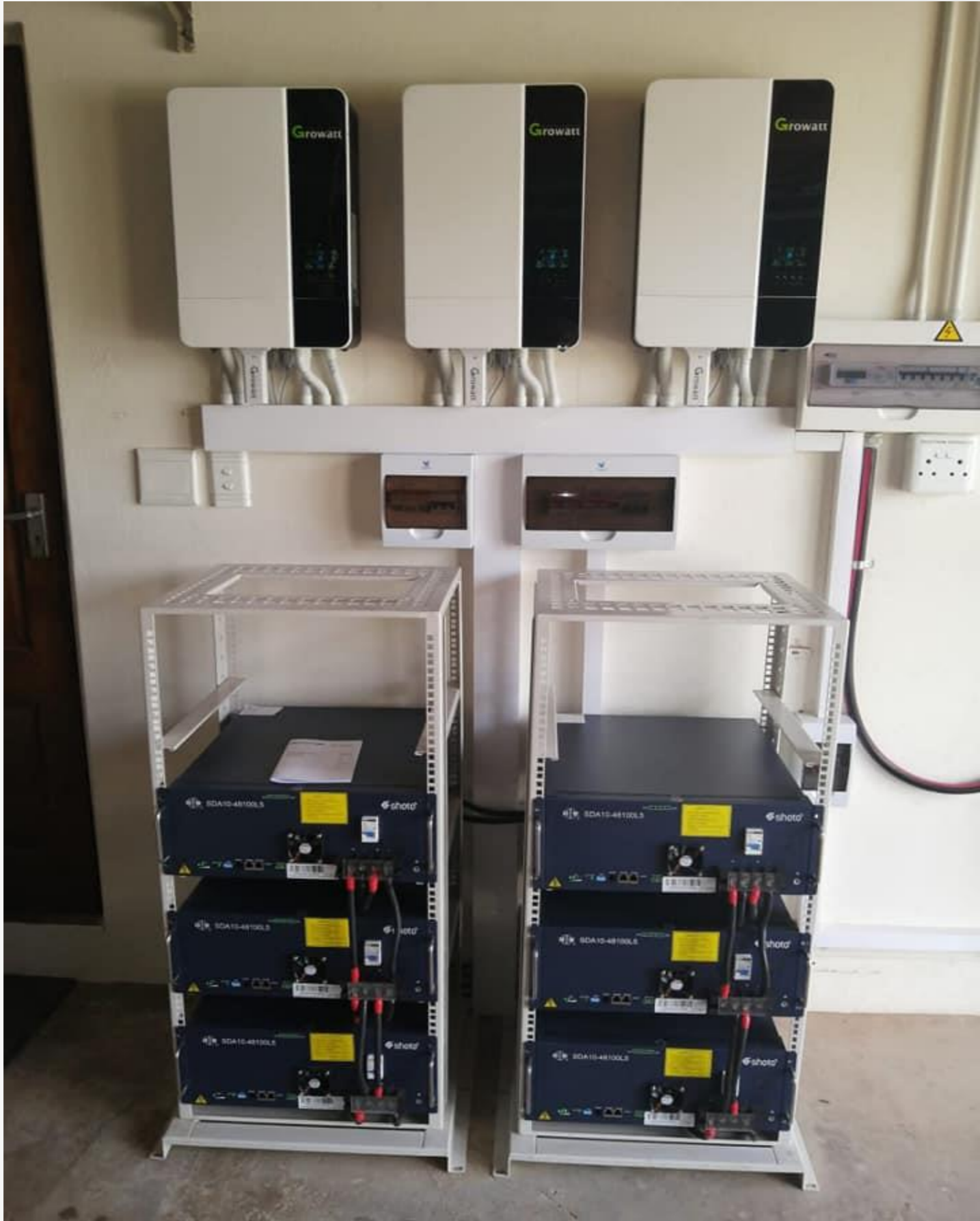
South Africa 15kW system
