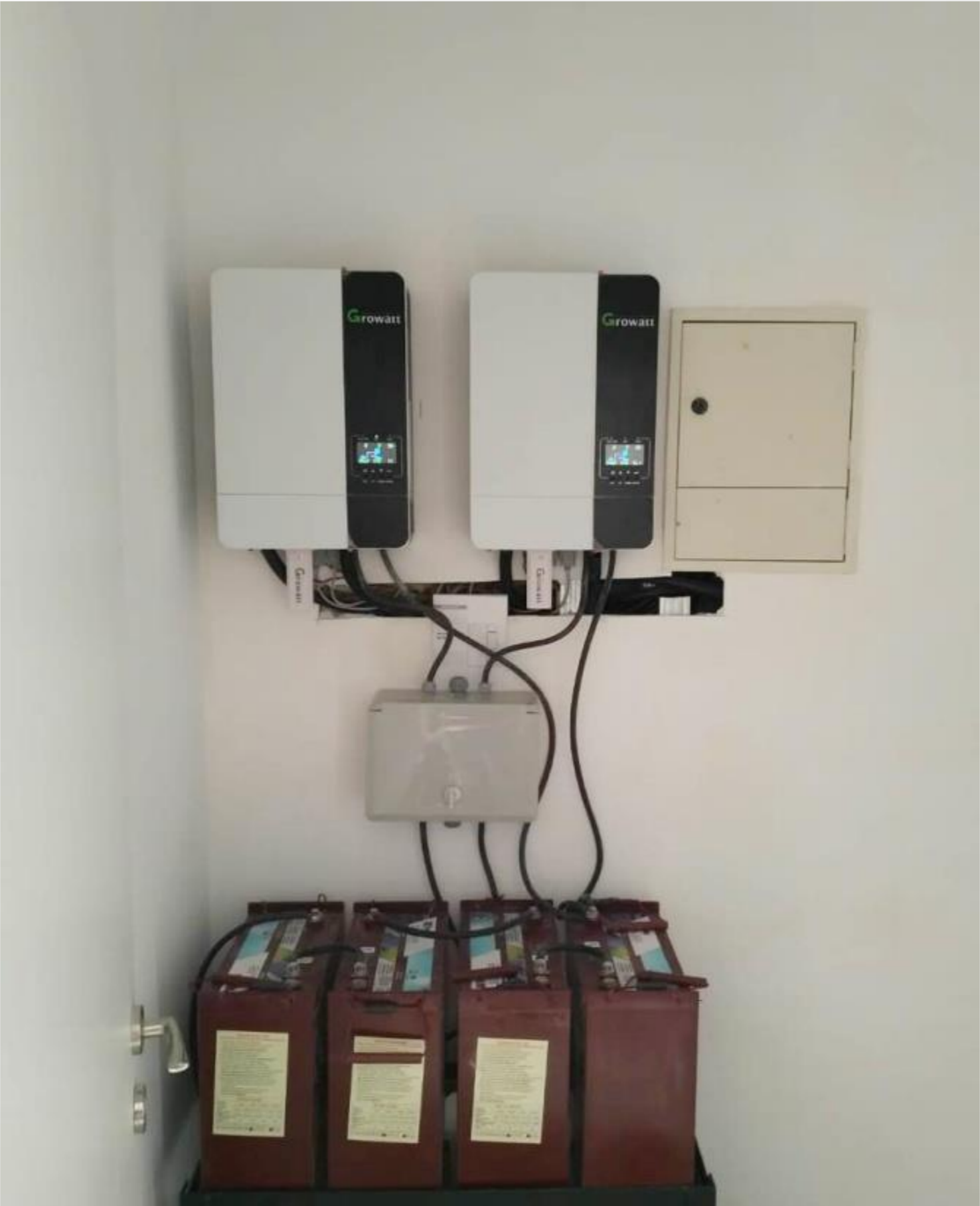
Turkey 10kW system
