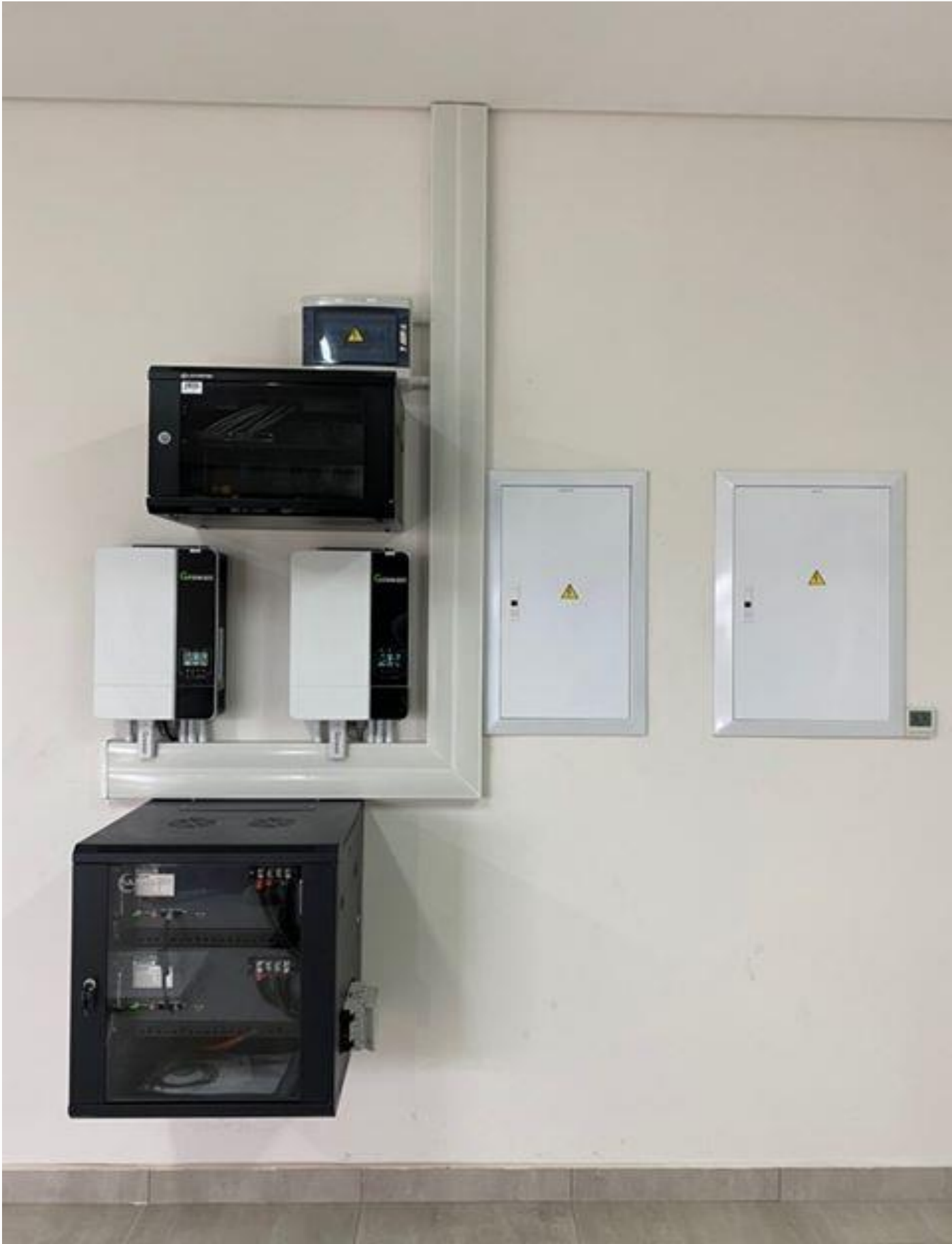
South Africa 10kW system
