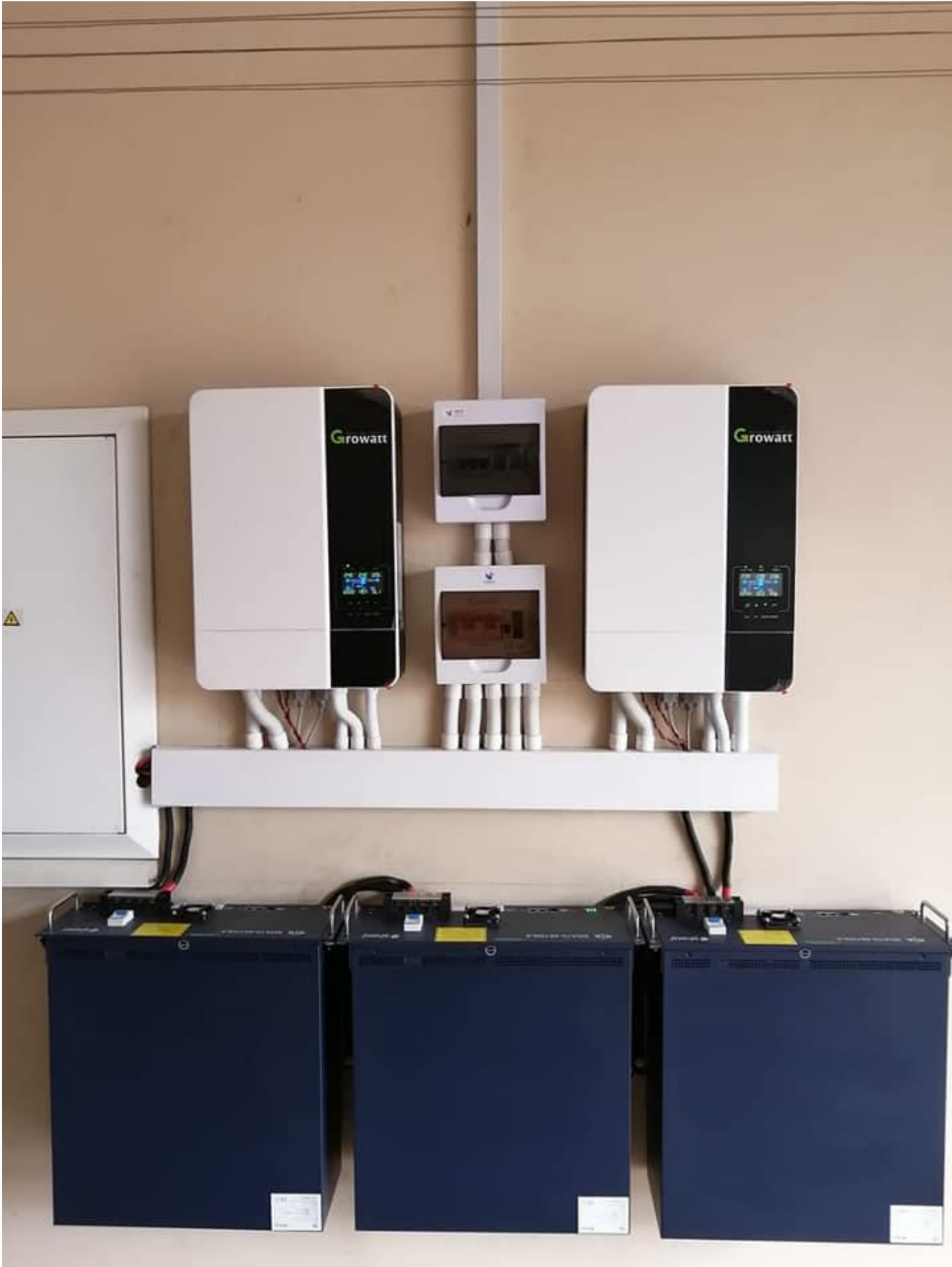
South Africa 10kW system
