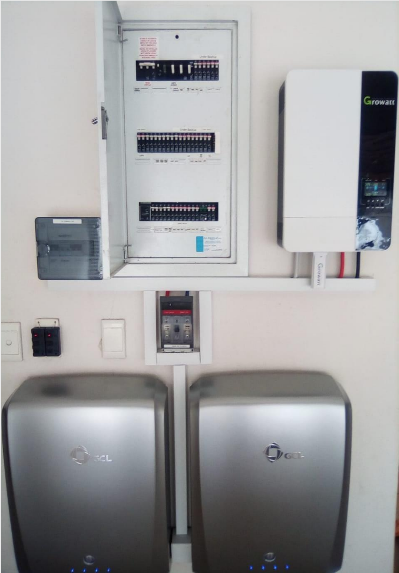
South Africa 5kW system
